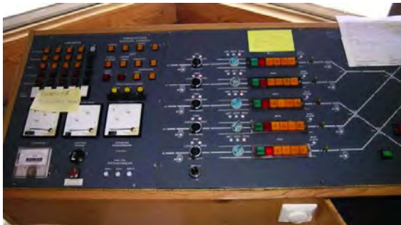
Figure 16: Control panel for brakes.
