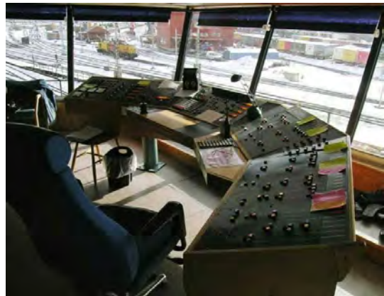
Figure 17: Work station for Westinghouse slip control system The control panel for the brakes to the left.
