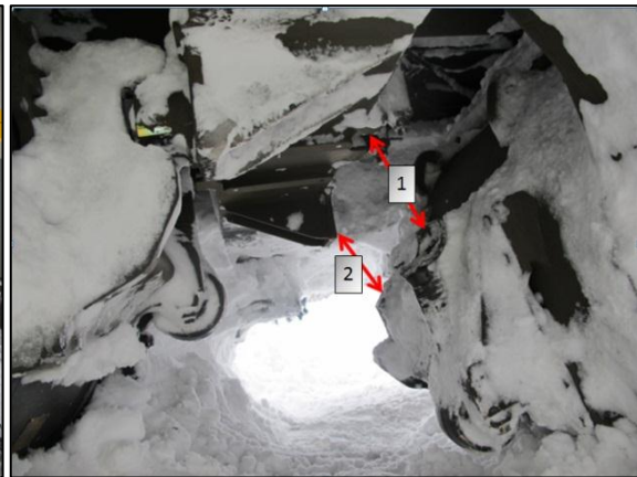
Figure 8: Broken torque link (1) and emergency support (2)
