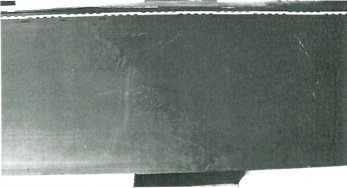
MRB upper surface 4.8. - 5.6. m away from the "zero line", seen towards the leading edge. Protective strip separation is noted locally.
