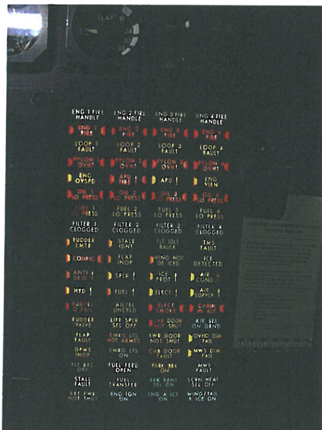
Figur 5.3, Master Warning Panel. (Light Test)
