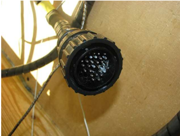
Picture 2 Signs of oxidation
