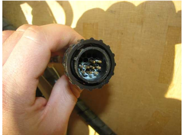
Picture 3 Signs of oxidation
