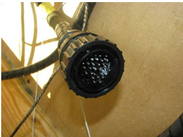
Picture 2 Signs of oxidation
