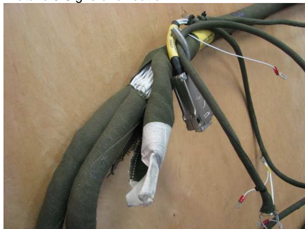
Picture 5 Damage of the loom
