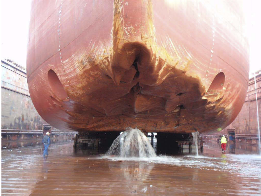
Figure 8: The picture is from the dry-dock in Gdansk and shows the ship seen from the front. The impression is from frame 200 and forwards. For the reader's information, the thruster tunnel is located between frames 211 and 241. In addition, there was damage to the longitudinal girders and shell plating at frame 116. About 130 tonnes of steel was replaced. Photo: DNV
