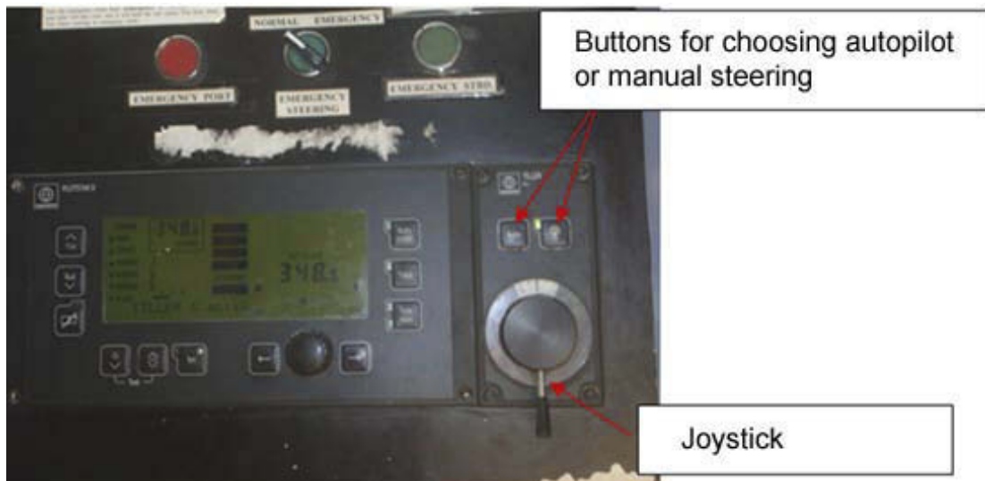
Figure 11: Autopilot located on the central manoeuvring console. A joystick can be seen at the right in the picture. A switch for changing from normal to emergency steering and buttons for emergency steering can be seen just above the autopilot consol.
