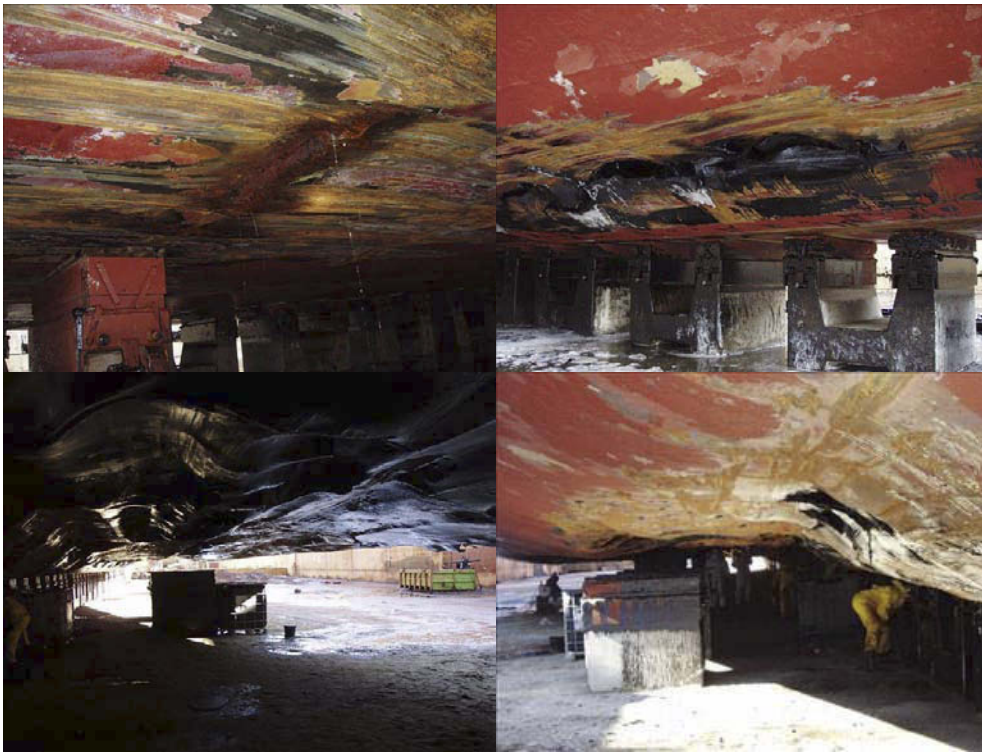
Figure 8: Godafoss under tow to the yard in Odense in Denmark, where DNV conducted the classification society's survey in the period between 5 March and 14 April 2011. All photos were taken by DNV while the vessel was undergoing repair.
