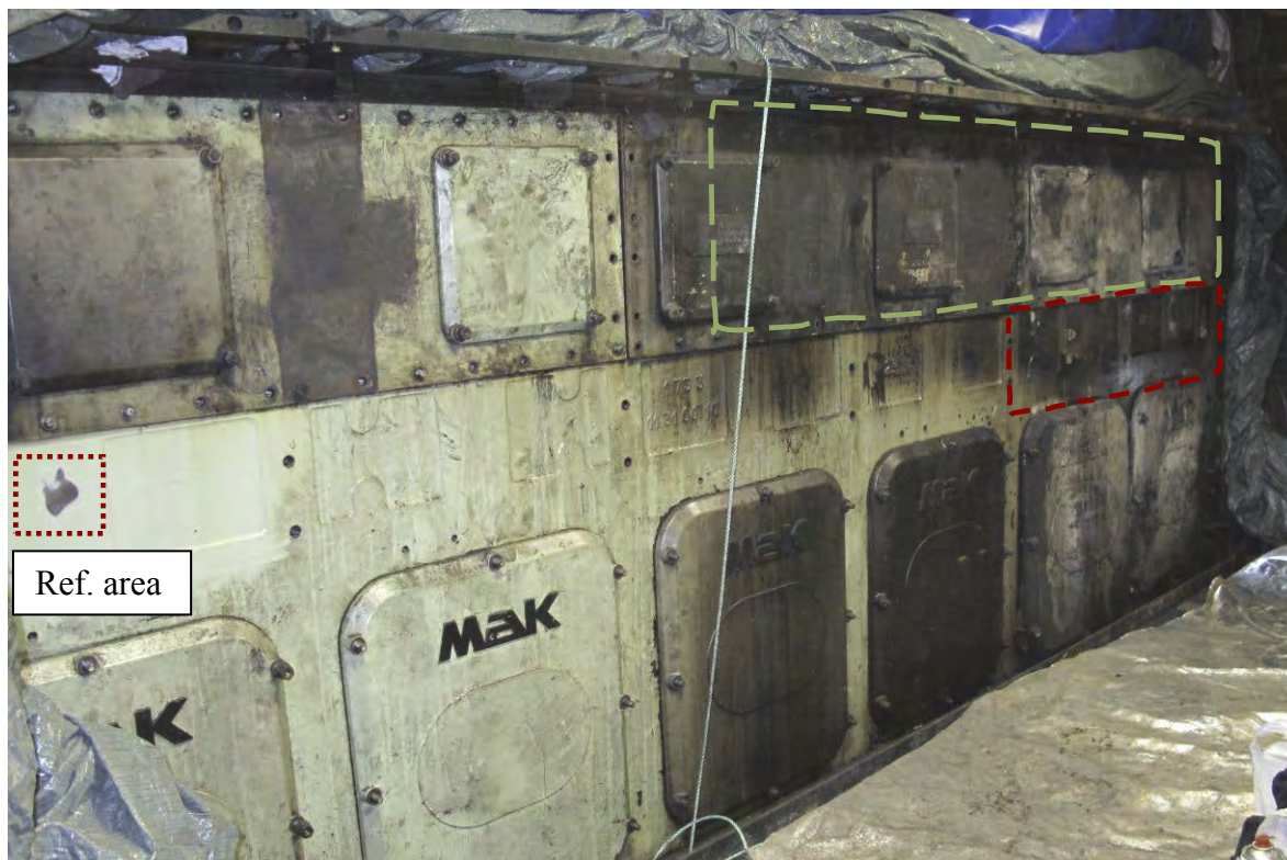
Fig. 1 Overview photo shows the heat affected areas (framed) on the stb. main engine on board the vessel M/S NORDLYS as observed by arrival. The green framed area is the hatch covers for the cam shaft consist of steel plates and hatch ways of aluminum alloy. The red frame indicates the part of the engine block which has suffered heat affection, see Fig. 2.
