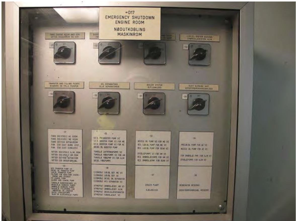
Figure 11: Panel for emergency shutdown of pumps, fans and engine room equipment. Photo: AIBN.
