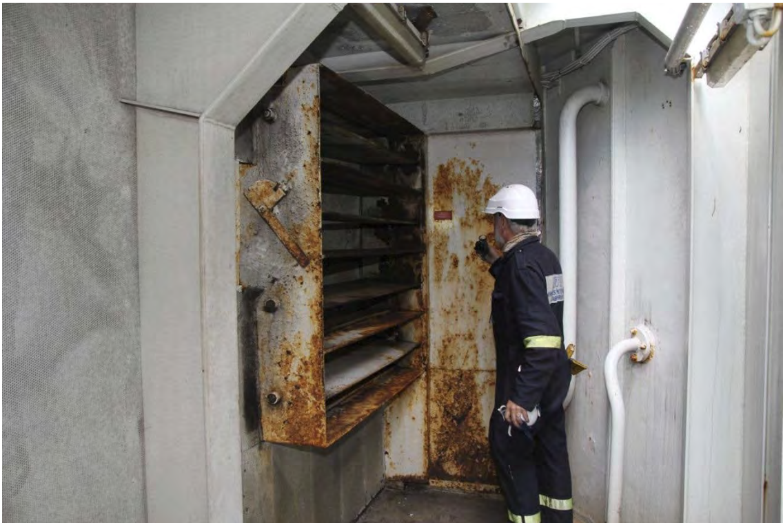
Figure 28: One of the dampers on the air inlet in the smokestack building on deck 7. Photo: SINTEF NBL.
