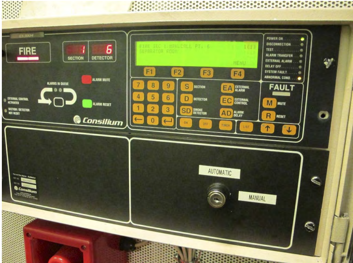
Figure 29: The photo shows the panel for the local application fire-extinguishing system. When the AIBN conducted its on board investigations, it was observed that the panel, which is located in the engine control room, was set to manual mode. There was no key in the switch for switching between manual and automatic extinguishing. Photo: AIBN.
