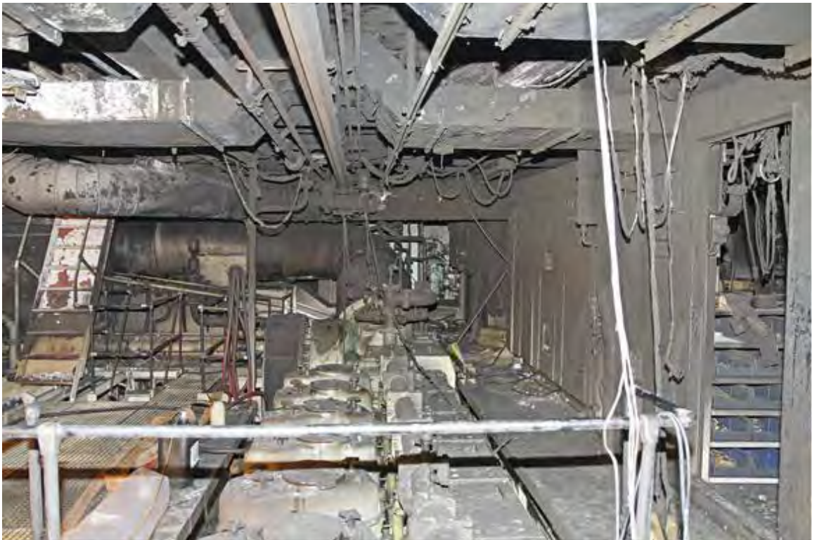
Figure 6: The port side of the main engine room looking aft from the forward gallery. The top of the port main engine is included in the photo. The door to the incinerator room can be seen on the right. Photo: The police.
