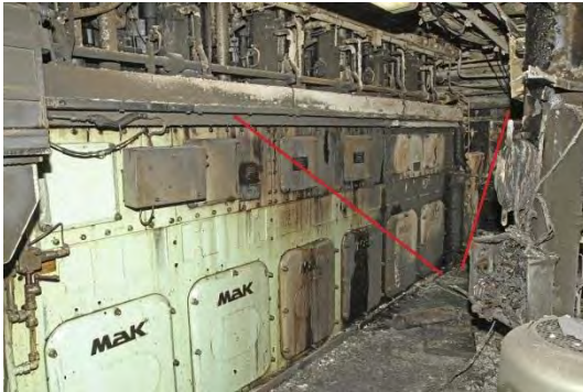
Figure 42: Looking forward along the starboard side of the starboard main engine at tank-top level. The fire has left a V-shaped mark from the floor upwards ('fire fan'). Photo: The police.
