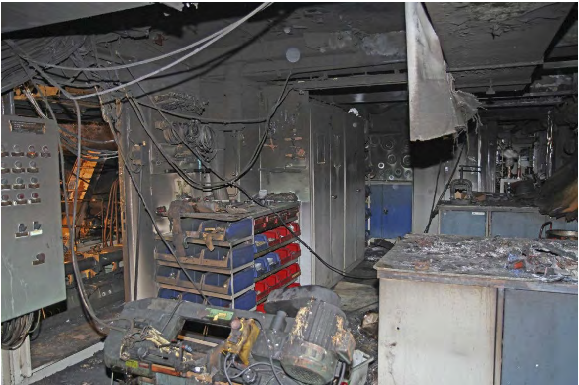
Figure 7: The interior of the incinerator room where the chief engineer came from when he met the motorman in the separator room. Photo: The police.
