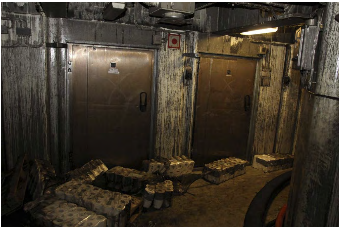
Figure 8: Outside the cold provision stores between the midship stairwell and the main engine room on deck 1. The temperature was so high that it melted the plastic wrapping around the toilet paper rolls. Photo: SINTEF NBL.
