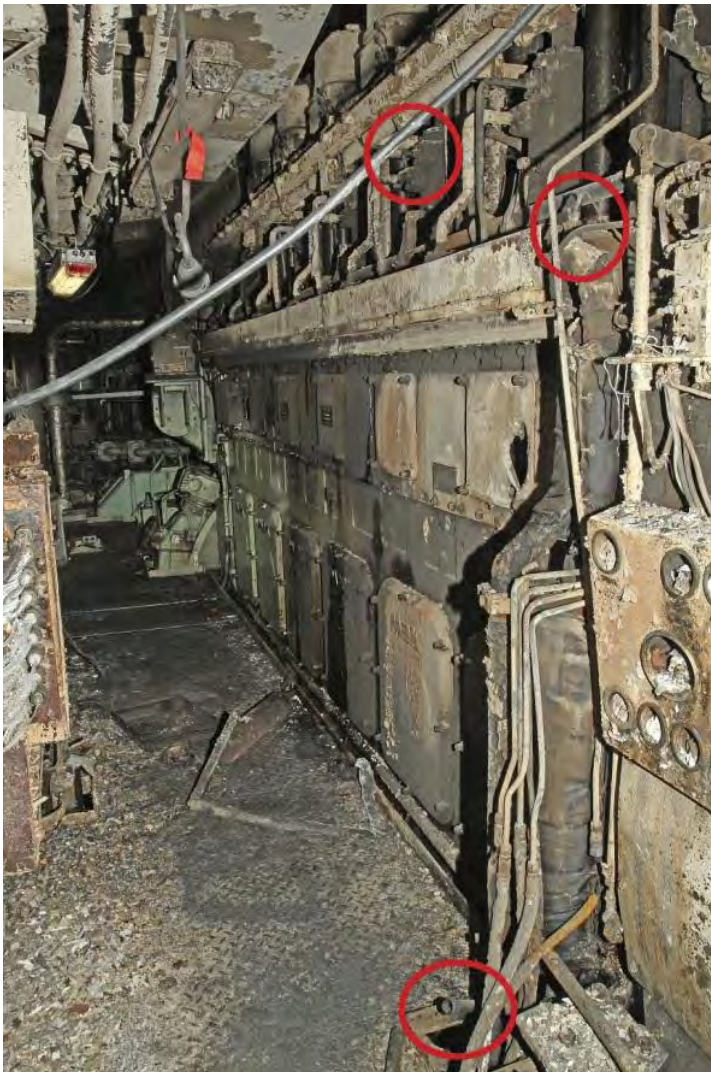
Figure 45: Position of the temperature sensor, ringed in at the top right of the photo, on top of the fuel rack. In other words, the sensor was placed in the immediate vicinity of both leakage points, ringed in at the top and bottom of the photo, respectively. Photo: The police.
