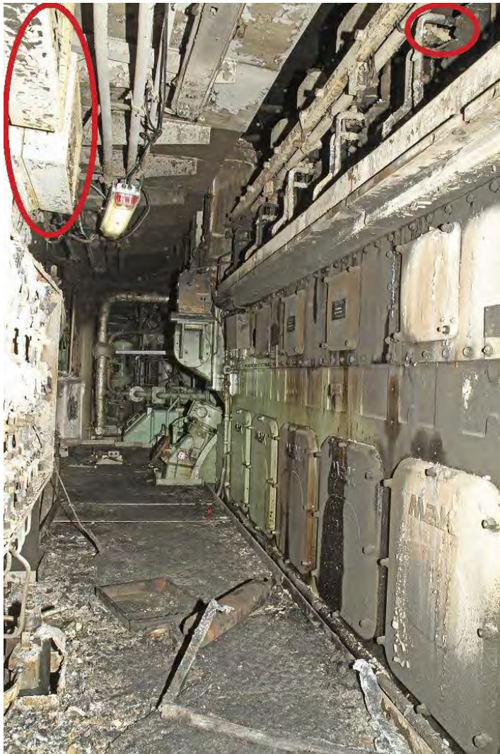
Figure 46: The SAU8 and SAU12 control cabinets, ringed at the top left of the photo, were at a horizontal distance of about one metre from the leakage at fuel injector pump no 5, ringed in at the top right of the photo. Photo: The police.
