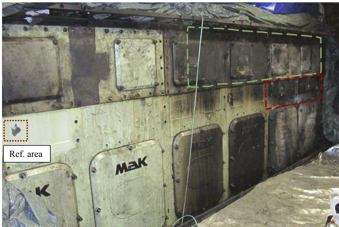
Fig. 1 Overview photo shows the heat affected areas (framed) on the stb. main engine on board the vessel M/S NORDLYS as observed by arrival. The green framed area is the hatch covers for the cam shaft consist of steel plates and hatch ways of aluminum alloy. The red frame indicates the part of the engine block which has suffered heat affection, see Fig. 2.
