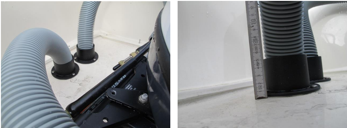
Figure 11: The arrangement for the cables and the fuel supply line for the motor. Photo: AIBN
