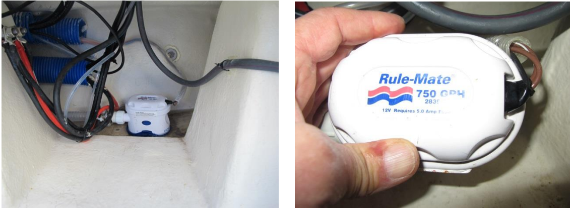
Figure 5: 'Viking 7' was arranged with a bilge pump at the stern below the inner liner. Photo: AIBN
