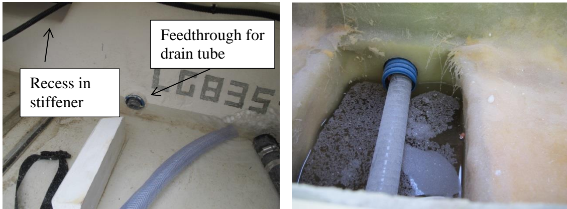
Figure 18: The photo on the left shows the unsealed feedthrough for the draining tube from the wheelhouse viewed from abaft, i.e. from the space below the flush hatch in the inner liner. Part of a larger recess in the stiffener through which water could flow unimpeded from aft to fore below the inner liner can be seen in the upper left corner. The photo on the right shows the feedthrough for the draining tube from the wheelhouse viewed from the forward end, i.e. from the space below the wheelhouse. Photo: AIBN
