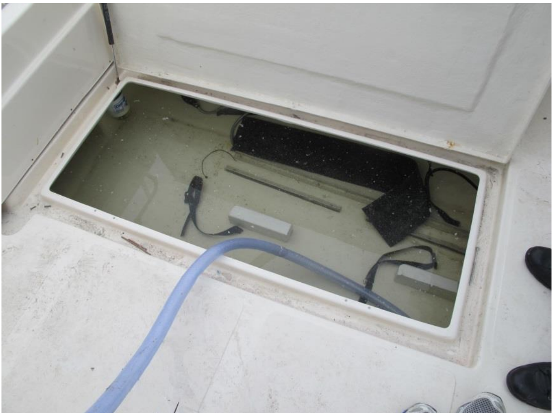
Figure 15: Filling the space below the inner liner through the flush hatch. The affixed fuel tank has been removed. Photo: AIBN
