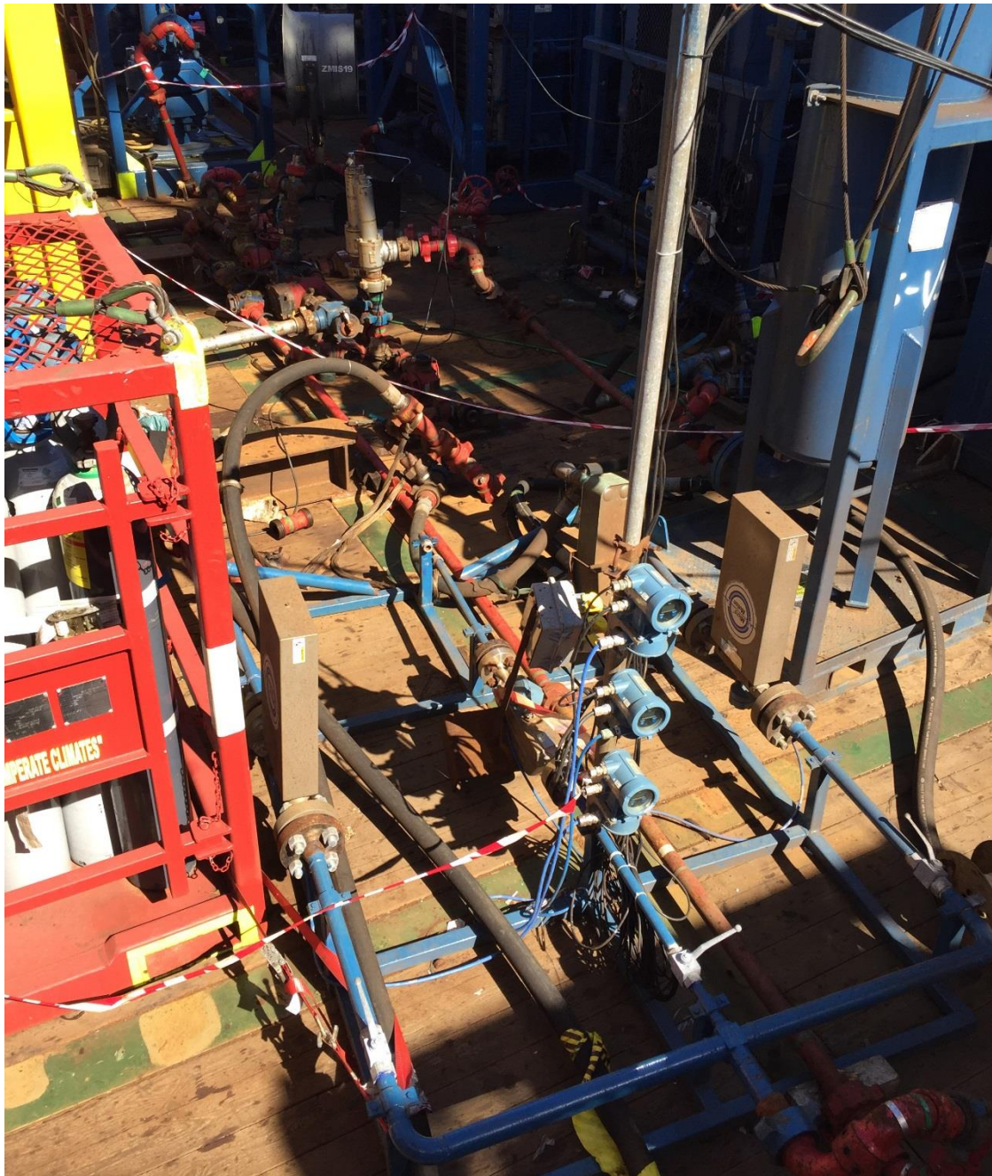
Figure 4: Pipes, hoses and valves placed between components on the open deck. Photo: The Brazilian Navy
