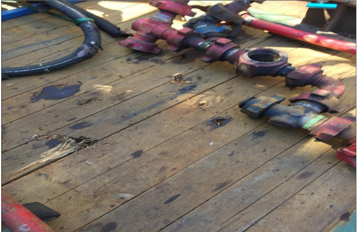
Photo 3: Pre-commissioning system equipment
