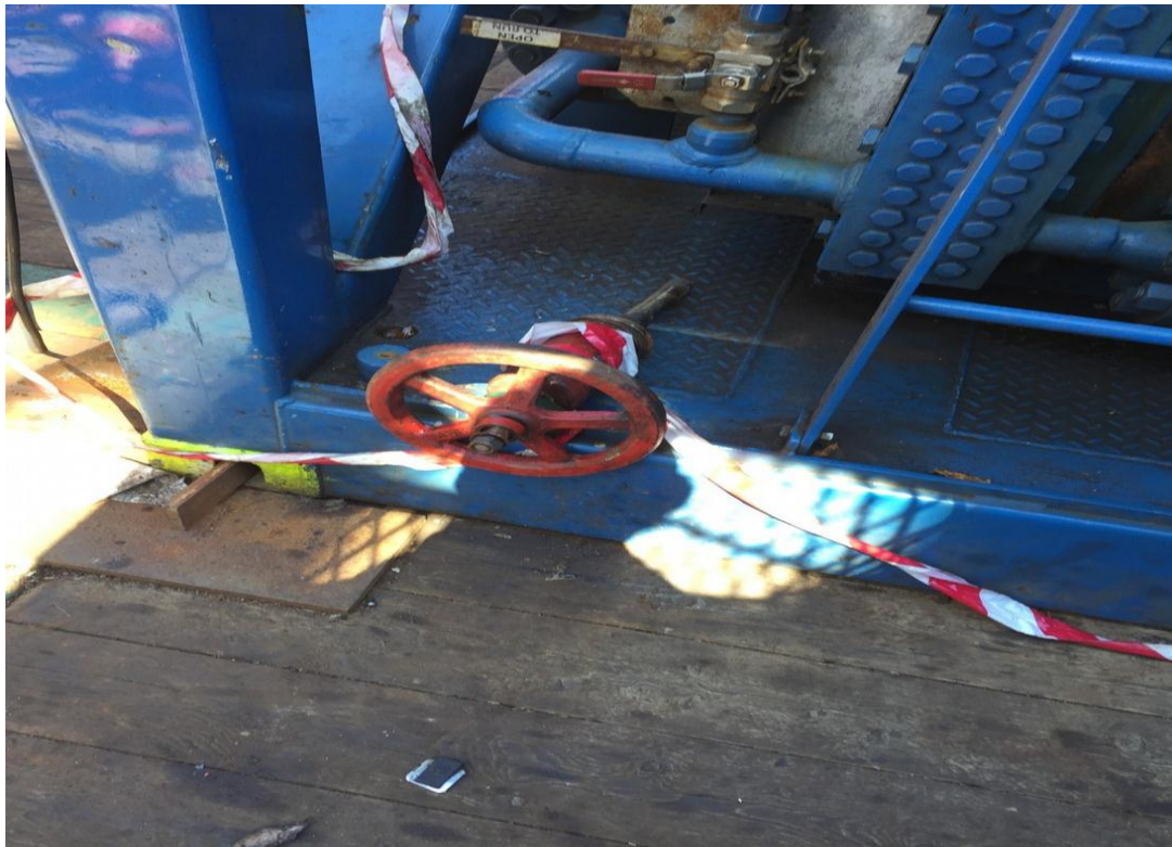
Photo 9: "Choke valve" failed
