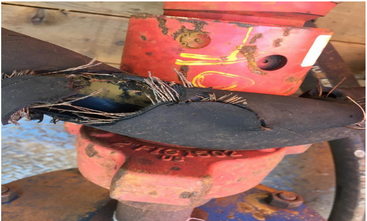
Photo 4: Faulty pre-commissioning system hoses
