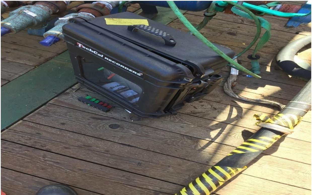
Photo 5: Pressure and temperature recorders not installed
