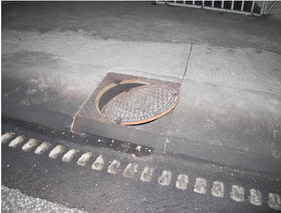
Figure 3: A surface water drain with an opening of 60 by 5 cm that faces the road surface. The black streak (roughly 0.7 m wide in Figure 3) on the road surface is where the greatest portion of the petrol flowed and was ignited (hence the marks). This surface water drain was 187 m down-slope from the trailer.
