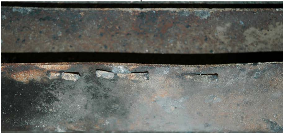
Figure 4 Image of trailer tongue end brace having spot welds and remains of wire mesh.
