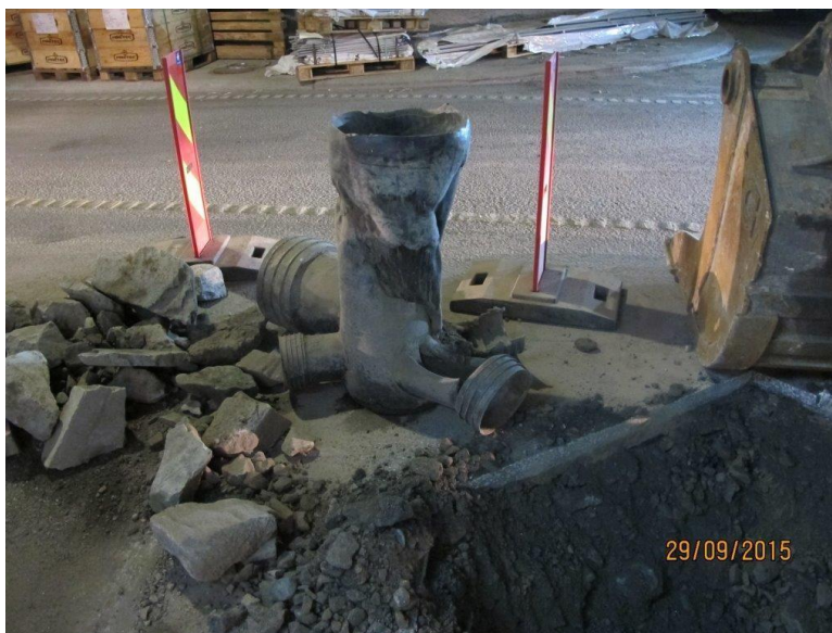
Figure 23: Parts of the rock water drain that was located outside the pumping station. The signs of an intense fire are quite clear.
