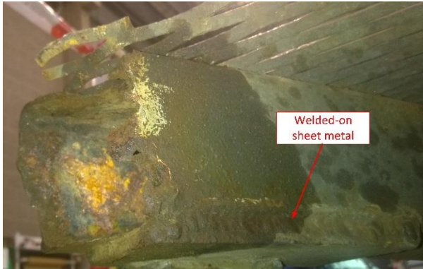
Figure 15: Sheet metal welded onto the left drawbar rod during repair work. Photo: AIBN
