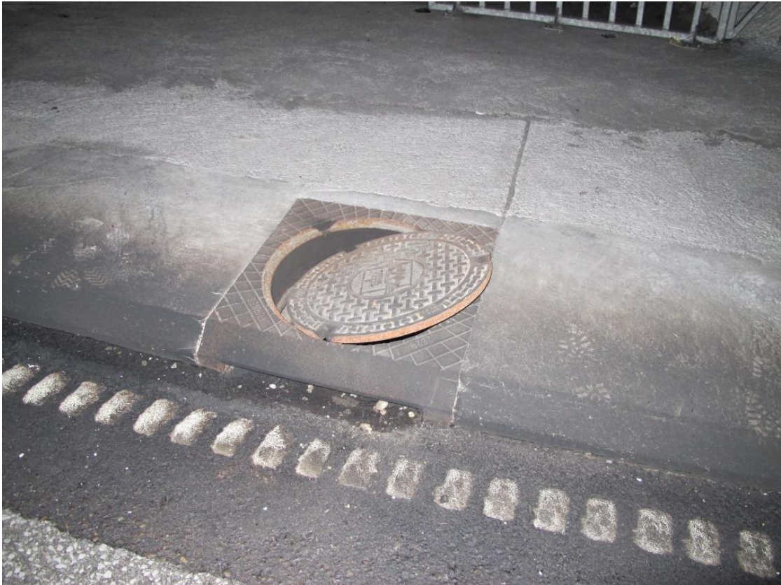
Figure 30: Sand trap with gully approximately 270 metres below the scene of the fire. The photo shows dark marks caused by petrol running past the gully. Photo: AIBN
