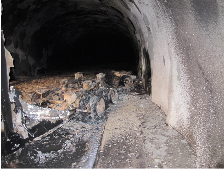
Figure 2: The position of the trailer after the fire. Note that the front wheels are directed towards, and in close proximity to, the wall.
