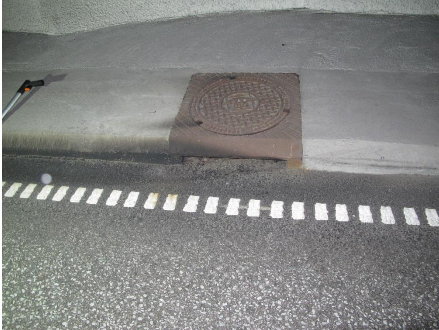
Figure 4: Photograph showing Drain 1, which was furthest down the slope, and which is also visible in Figure 3. Here, the evidence suggests that petrol flowed into, rather than past, the drain. This petrol is calculated to have reached the drain roughly 25 seconds after the start of the fire (3 minutes after the incident occurred); the flame front did so roughly 2 minutes after the start of the fire.
