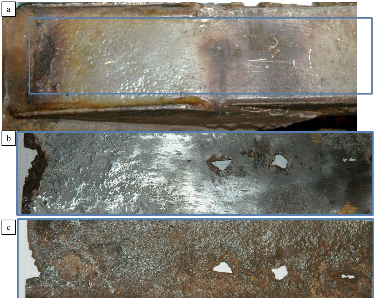
Figure 7a: Image showing area selected for characterization of the general corrosion. b: Image of the outside following paint removal. c: Image of inside following removal of corrosion products.
