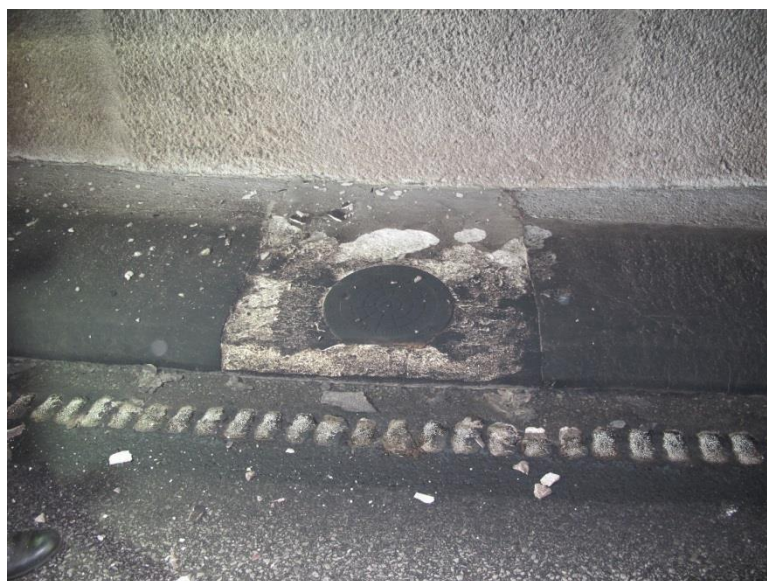
Figure 22: An inspection hatch, located 175 m from the pumping station and belonging to the rock water drainage system.
