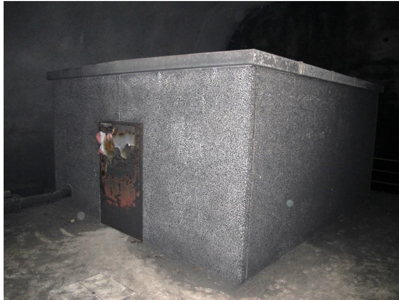
Figure 21: Very marked fire damage on the door of the pumping station, located directly above the sludge basin. Just past the pumping station was a grated floor, which was above the sludge and water basins. There were clear signs of a fire having occurred in the sludge basin.
