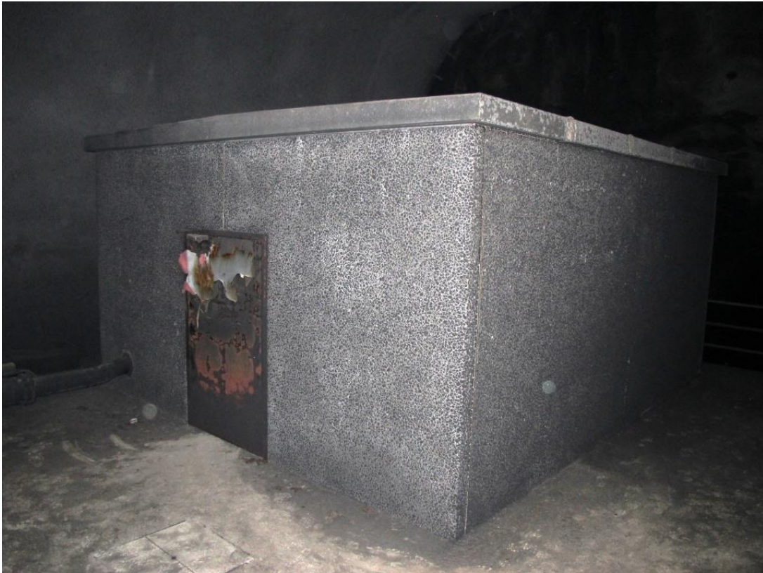
Figure 31: The pumping station at the bottom of the tunnel with fire and soot damage to the surfaces. Photo: AIBN
