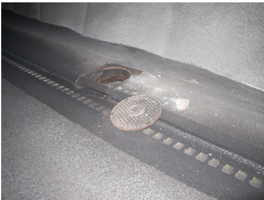
Figure 1: A photograph showing how petrol flowed on the surface of the road, from the trailer and down-slope towards the pumping station at the bottom of the tunnel. The dark section of the road surface shows where the petrol flowed and subsequently burned. The drain cover had a diameter of 0.609 m.
