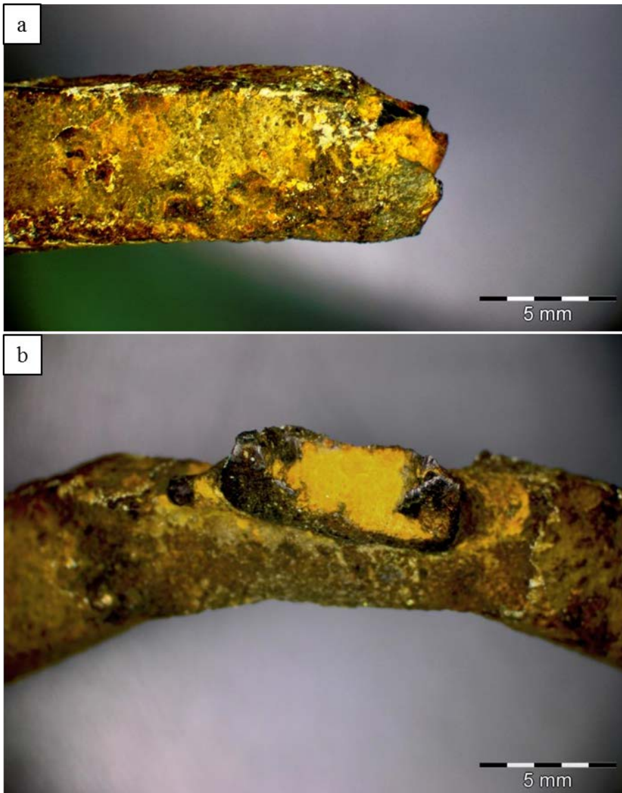
Figure 17 Image of a: failed wire in wire mesh and b: failed spot weld.
