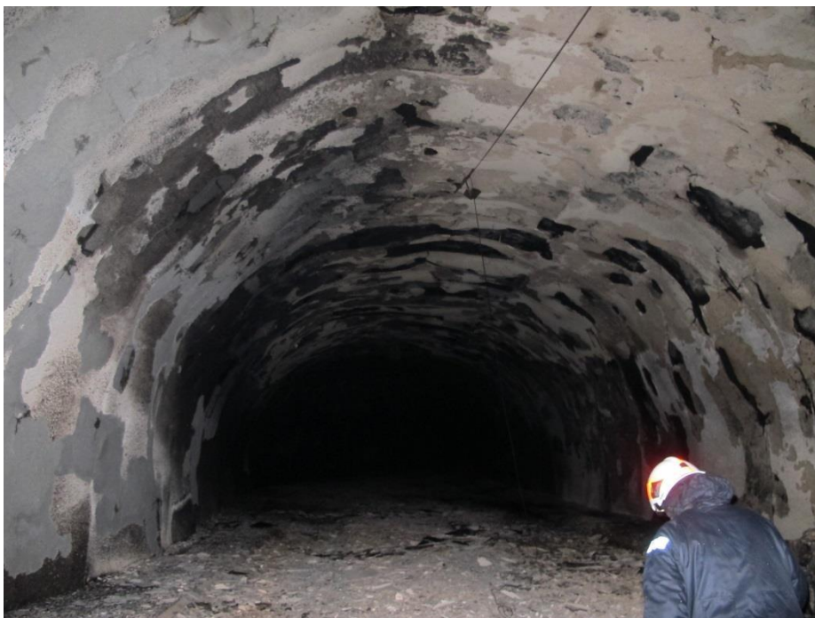
Figure 17: Damage to the shotcrete just up-slope from the trailer.
