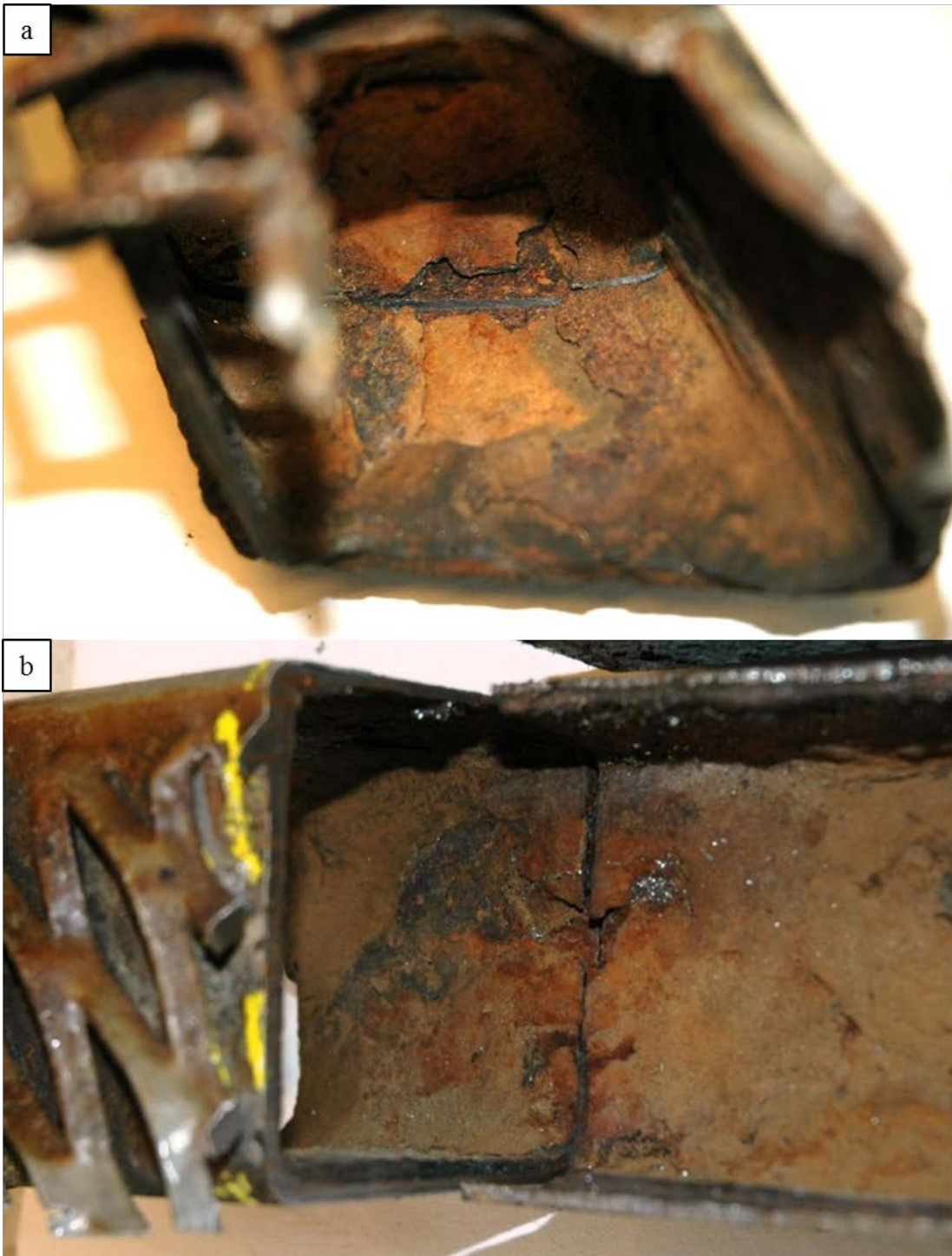
Figure 6 a: Image of through wall thickness corrosion at right side (H), b: Image of through wall thickness corrosion at left side (V).
