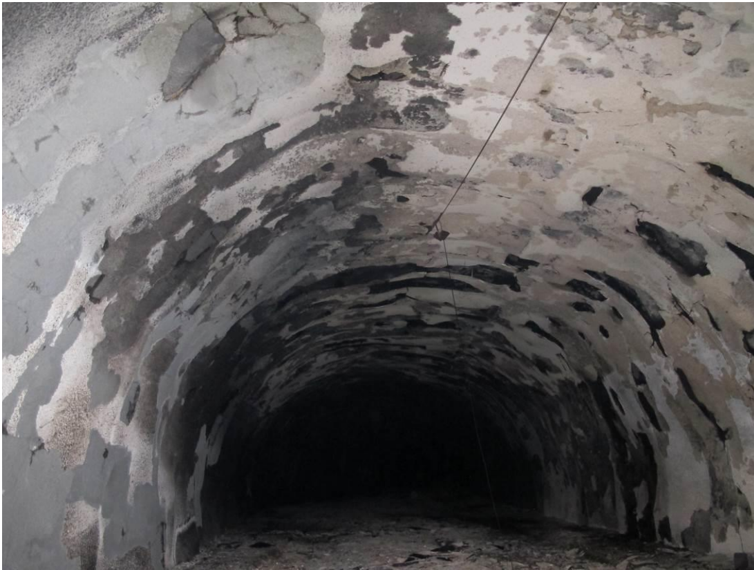
Figure 9: Shows damage to the tunnel bore in the area of the tank trailer, viewed in the direction towards which the smoke was ventilated. Photo: AIBN
