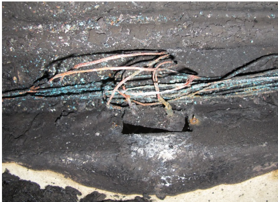
Figure 10: Licence plate light from the fire on 17 December 2016 with arcing damage to the circuit. Photo: AIBN
