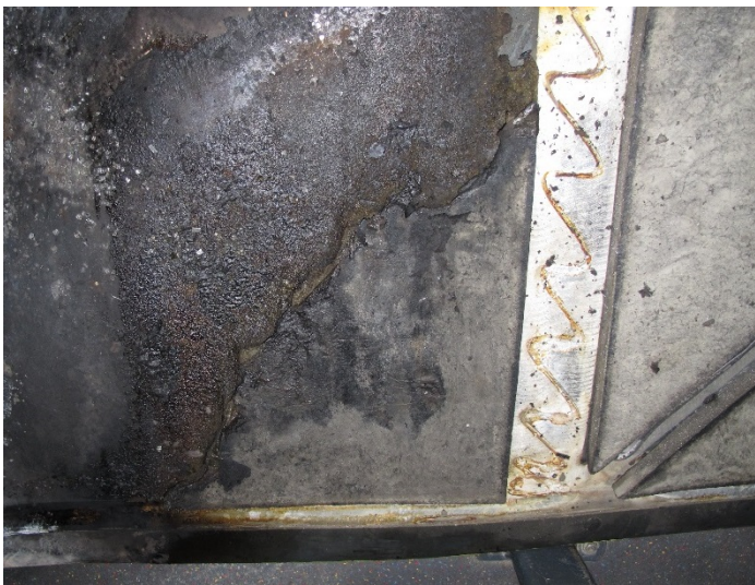
Figure 15: Right side of the V-shaped burn in the insulation on the rear hatch on 17 December 2016. Photo: AIBN
