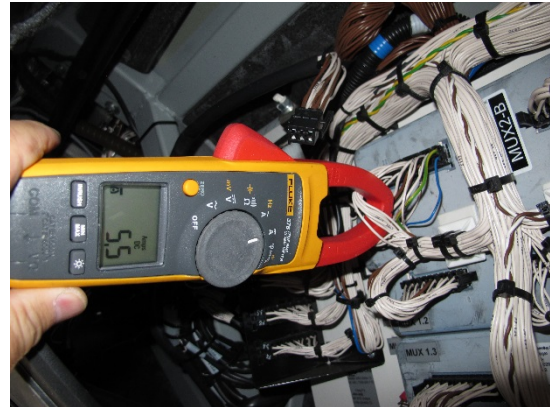
Figure 18: The licence plate lighting circuit at 5.5 A, more than the consumption at the time of the fire in the licence plate light. Photo: AIBN
