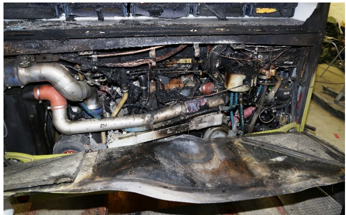
Figure 7: From the fire on 17 December 2016. Melted plastic in the engine compartment and insulation burnt in a V shape on the inside of the rear hatch. Photo: The police
