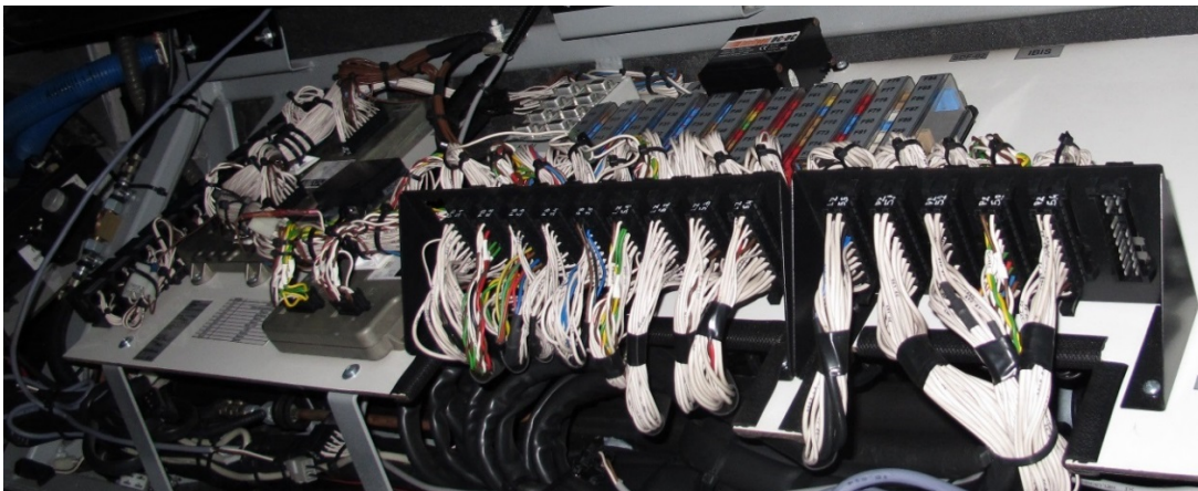
Figure 12: Fuse box, multiplexers and wiring in the buses in question. Photo: AIBN
