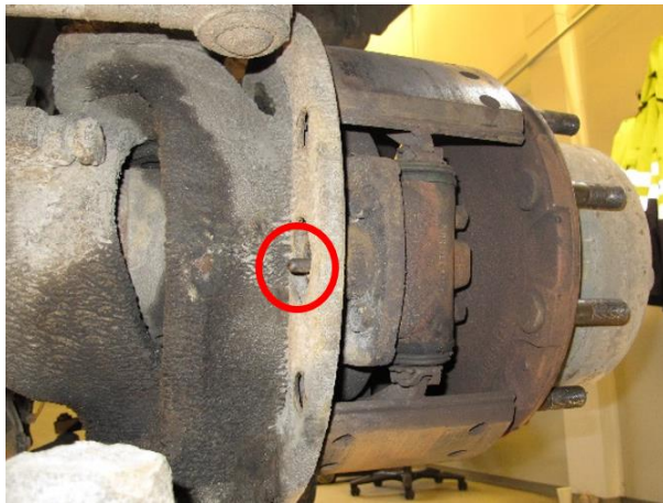
Figure 5: Push rod stuck inside the wheel cylinder on the left side. Wheel cylinder and brake shoe on the left side. Photo: AIBN
