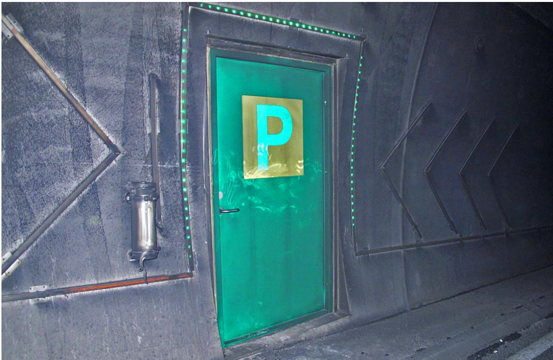
Figure 36: Dynamic green lights guide road users towards the emergency shelters. Arrows on the tunnel walls point the way to the doors of the emergency shelters. Photo: AIBN
