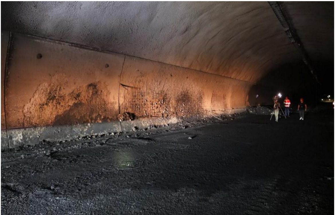
Figure 26: Spalling damage to wall elements inside the tunnel. Photo: Aas-Jakobsen/NPRA
