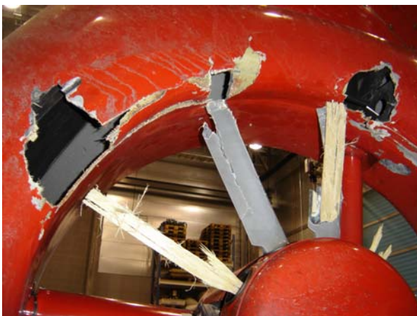
Figure 8: Damage to blades and the tunnel.
