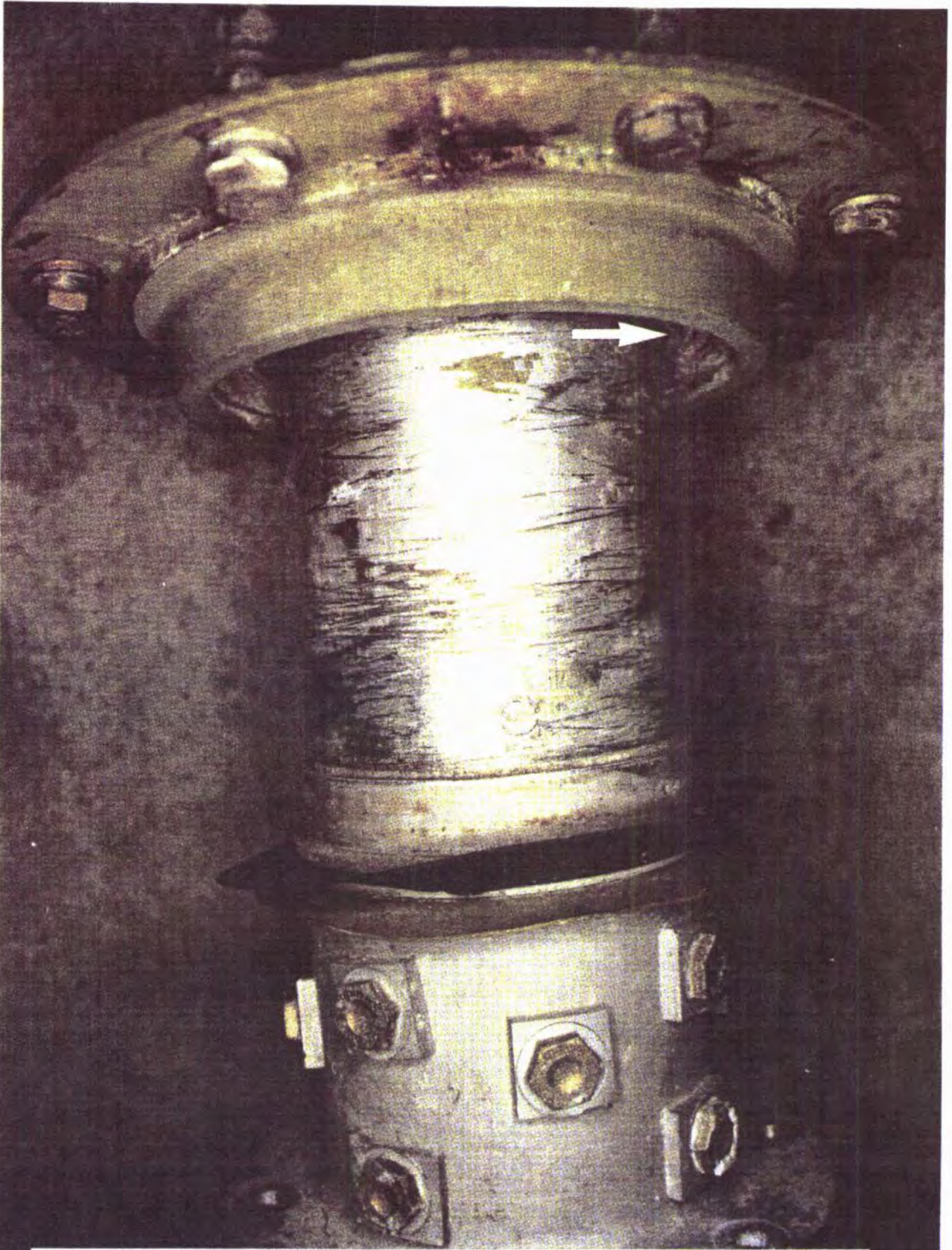
PHOTO 13 Fully displaced (outboard) retainer collar reveals 3" zone of severe scoring on torque tube. The scoring was caused by abnormal rotation of the retainer collar inner land (arrow) against the tube.
