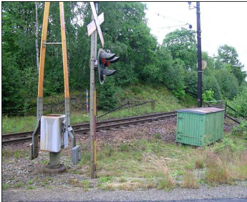
Figure 55: Example of a cabin that does not block any sight lines (Sweden).
