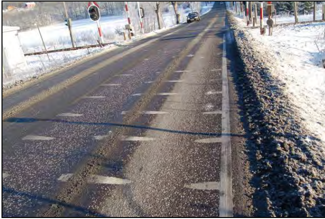
Figure 50: Example of poorly maintained rumble strips (Tomsbakken LC).
